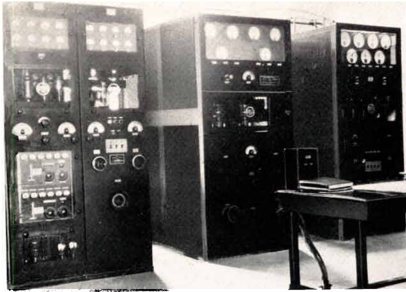
FIGURE 3—THE 10 KW RCA VICTOR TRANSMITTER STATION CP3
